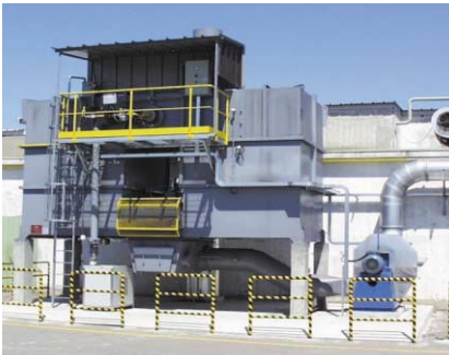
Exhaust gas combustion equipment at YKK Italia
