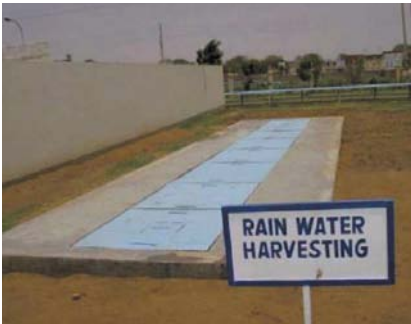
Rainwater harvesting equipment at YKK India
