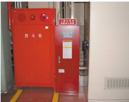
Fire extinguishing equipment for duct fire prevention (center)
