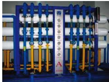
Recycling of wastewater at plants
