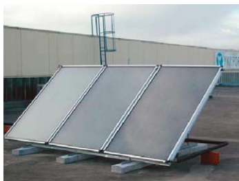
Solar heat panel
