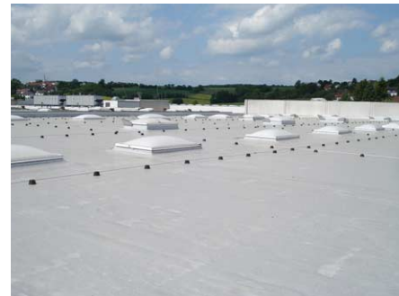
YKK DEUTSCHLAND GMBH We installed insulation on the roof of the plant which allowed us to reduce the amount of natural gas used for heating by 10%.
