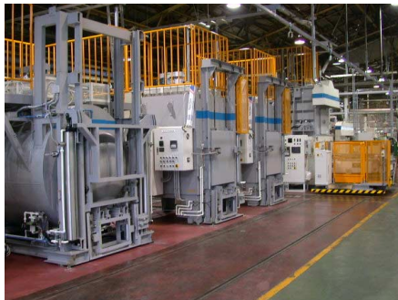
YKK Corporation Machinery and Engineering Group By changing the quenching method used on the heat treatment line, we were able to achieve an annual reduction in CO 2 emissions of 125 tons.
